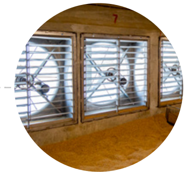
Large closed house with Evaporative Cooling System
