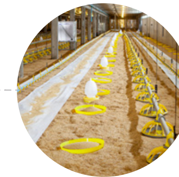
Automatic feeding and water system
